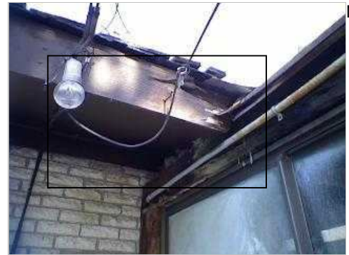
Water damage at the soffit area above the main disconnect.
